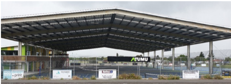
Masterton Netball Centre has a constructed cover with 5.5 metre sides and 7 metre peak. The centre report issues with the rain coming in the sides.
