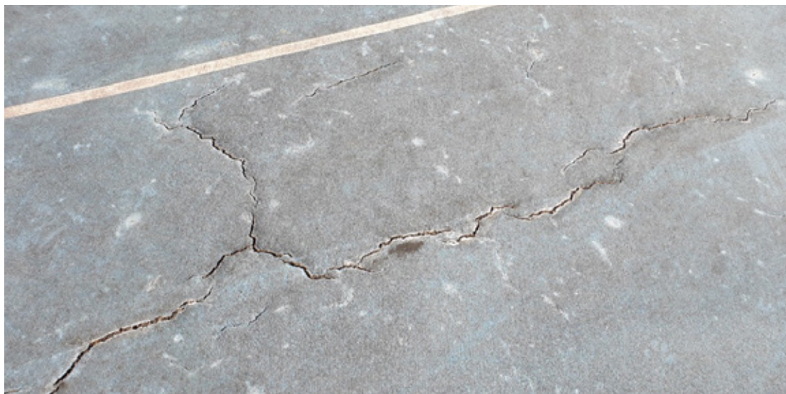
Netball court with extensive cracking, undulations, birdbaths, and discolouration. The indicative cause is poor drainage under the courts causing sub-structure movement resulting in structural cracks.
