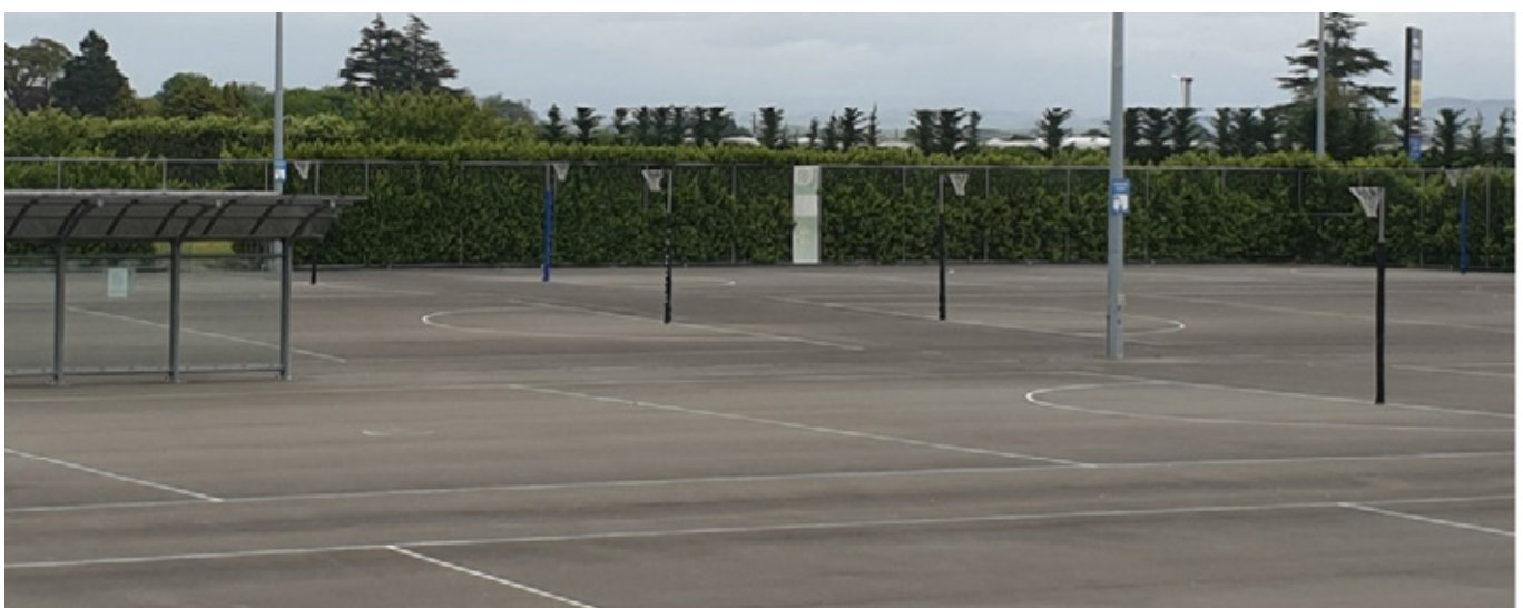
HAWKE'S BAY NETBALL CENTRE, MITRE 10 PARK WITH CROSS FALLS OF 1:90 AND LONGITUDINAL FALL APPROXIMATELY 1:500.
